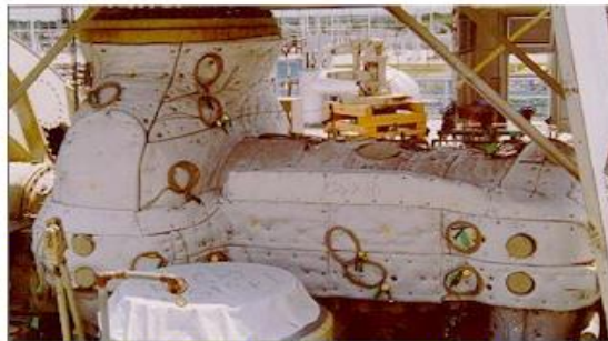
A turbine warming system installed on a steam turbine
